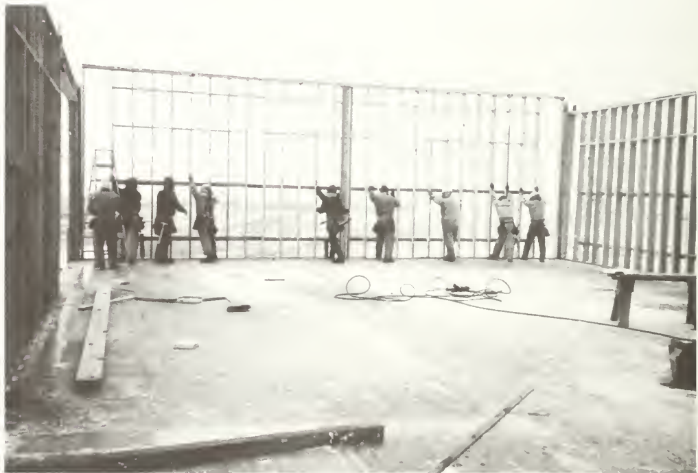
BLM engineers oversee construction of facilities such as this visitor center at Flagstaff Hills. Visitor centers and other recreation facilities promote tourism and help diversify local economies.
